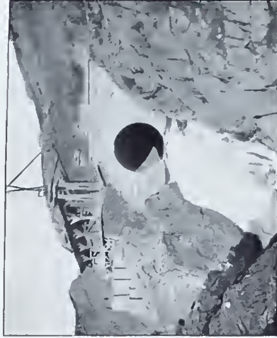
Craig Goch Culvert Outlet, Feb. 1898.
